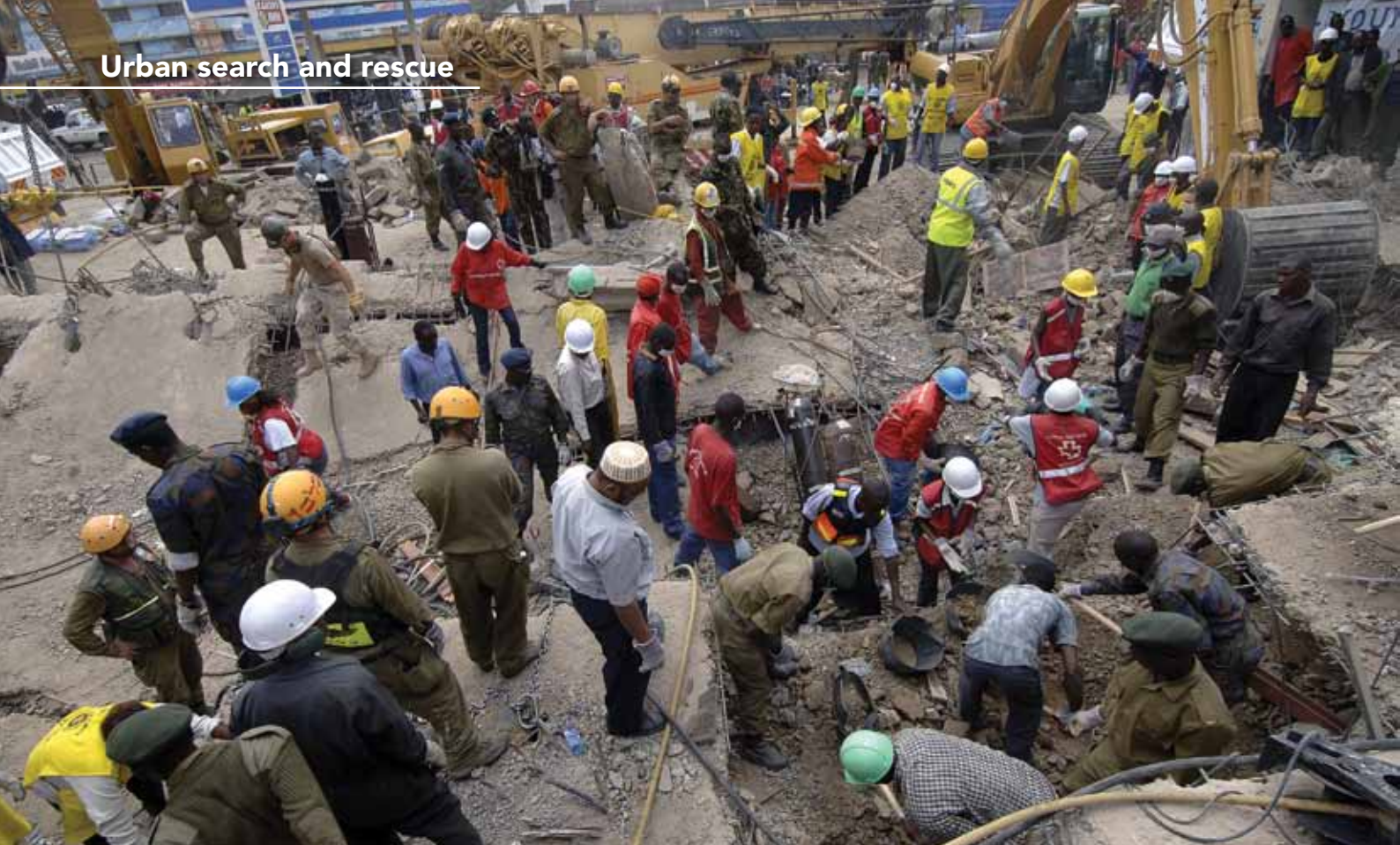
Volunteer workers dig for survivors in January 2006, after a building collapsed on Nairobi's Ronald Ngala Street in Kenya. US Air Force photo by Staff Sgt Ricky A Bloom
