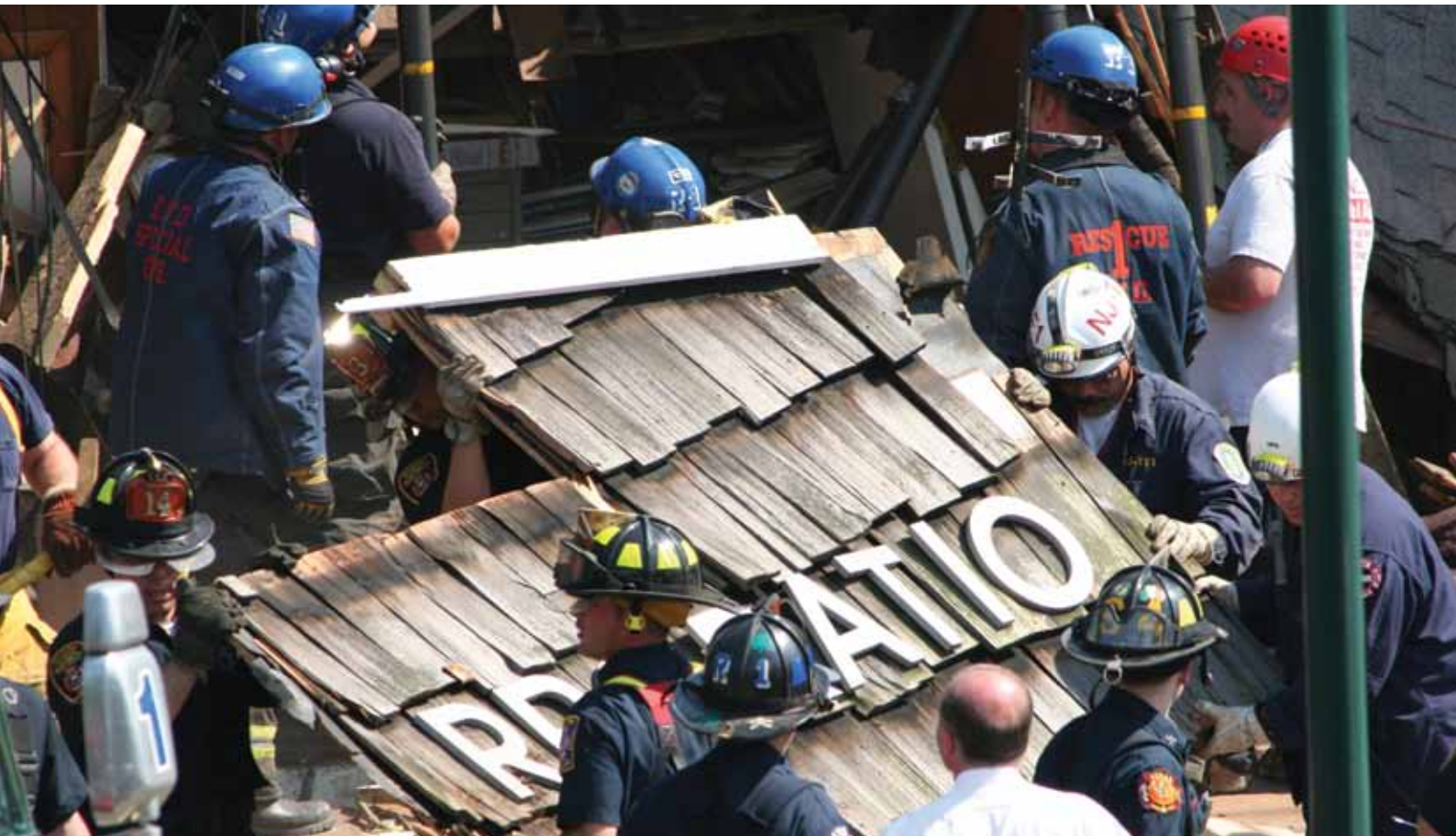
A building collapse in downtown Fanwood, New Jersey, USA
